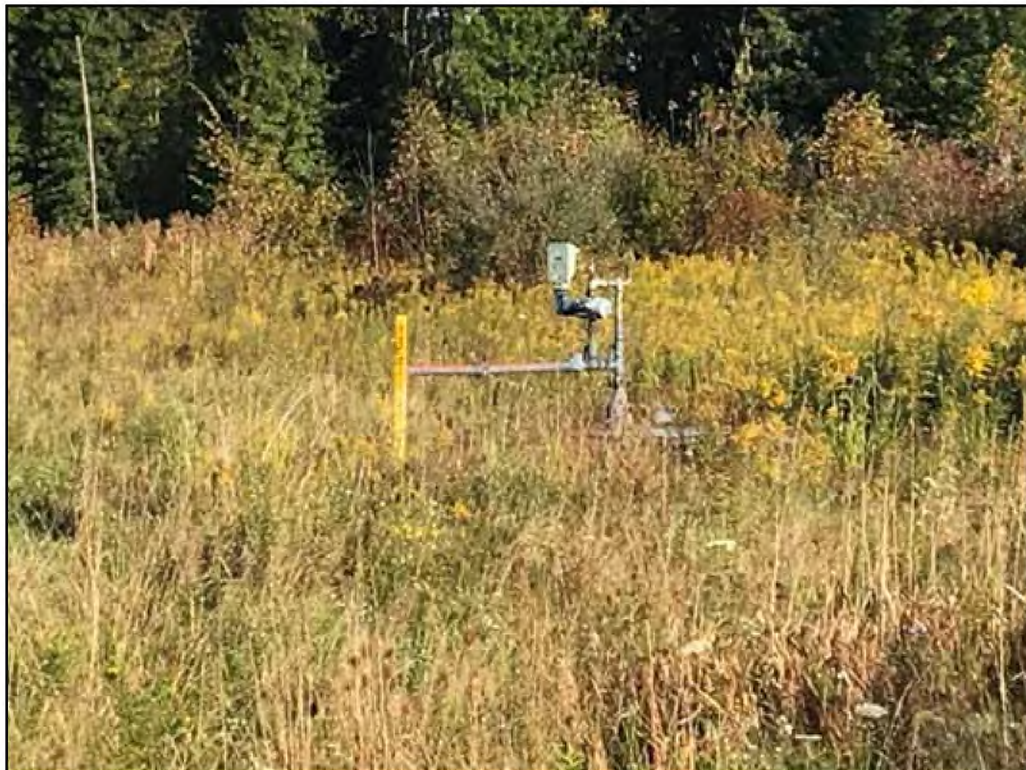
Photo 2: Gas meter in eastern portion of the Site.
