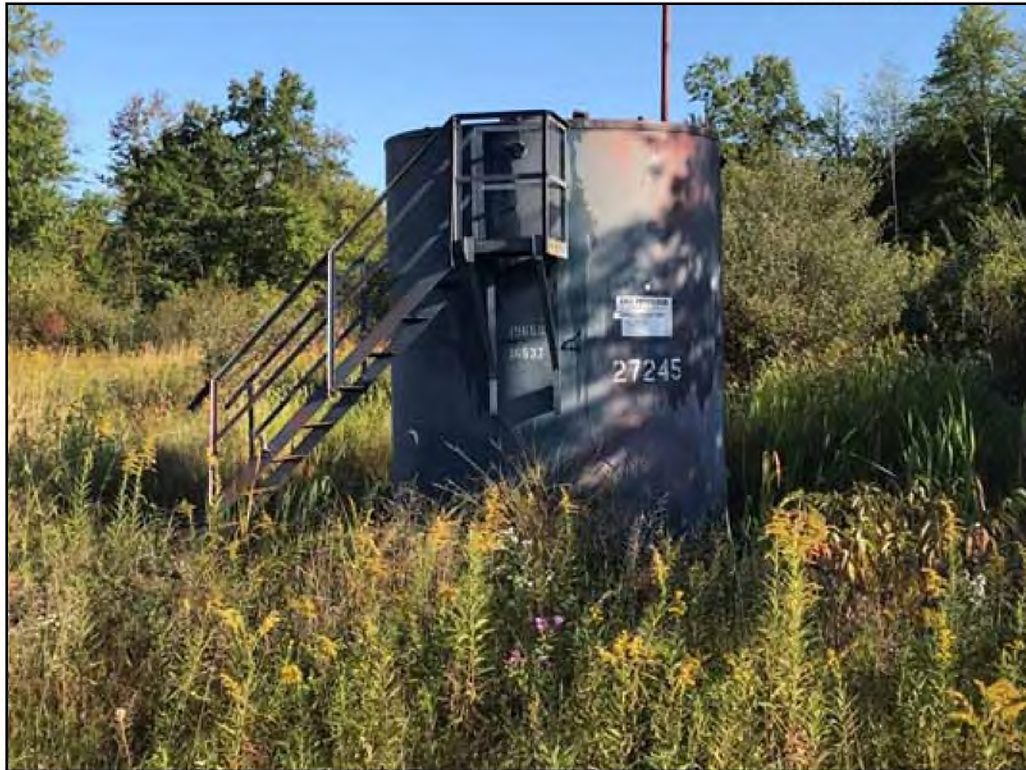
Photo 1: Looking north at oil collection tank in eastern portion of the Site.
