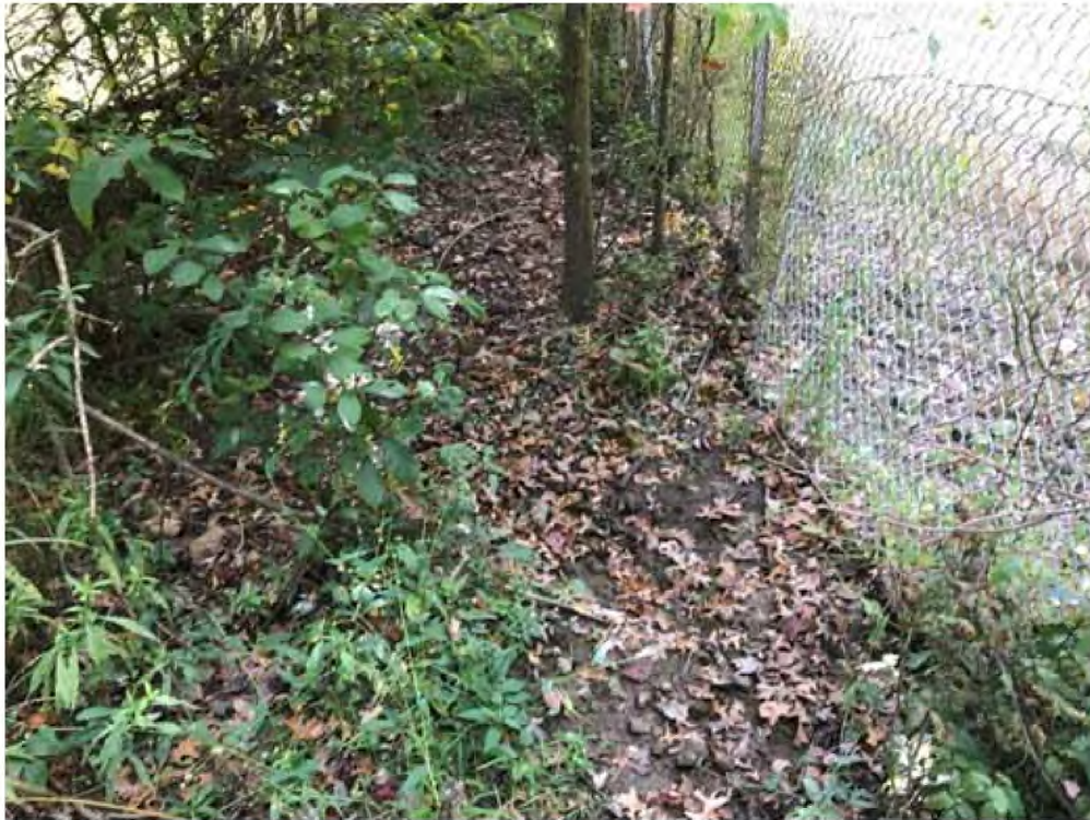
Photo 9: Small drainage feature along chain link fence on the western property boundary.
