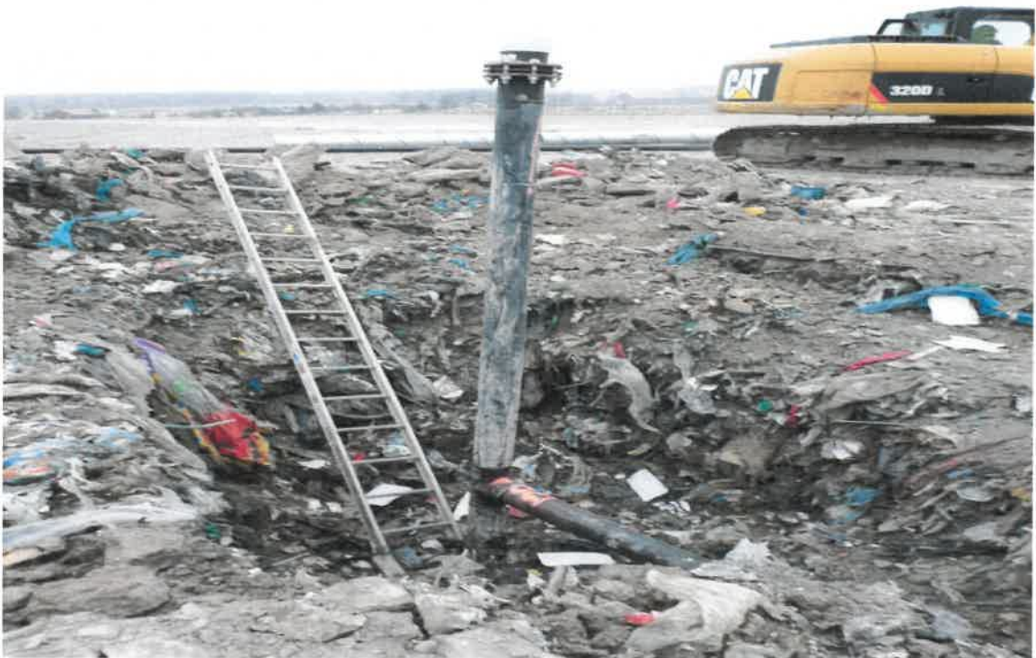
Photograph 18. 6" T connection at EW307R supplying vacuum to redrilled well EW303R, facing north.
