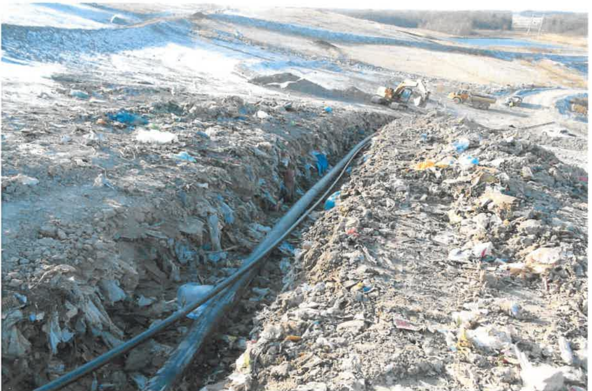
Photograph 6. 6" lateral, 2" air line from EW50R3 to 12" header, facing northwest.
