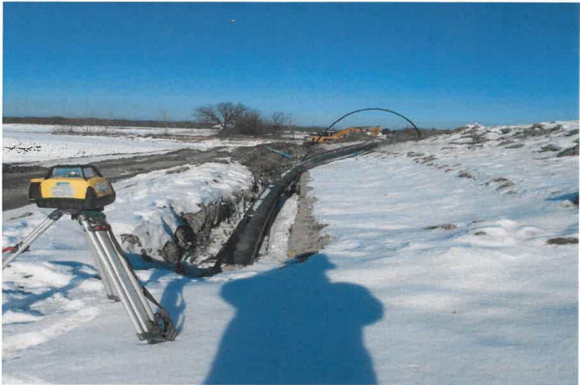
Photograph 11. Continuation of 12", 4", 2" to round the northwest corner near EW329, facing north.
