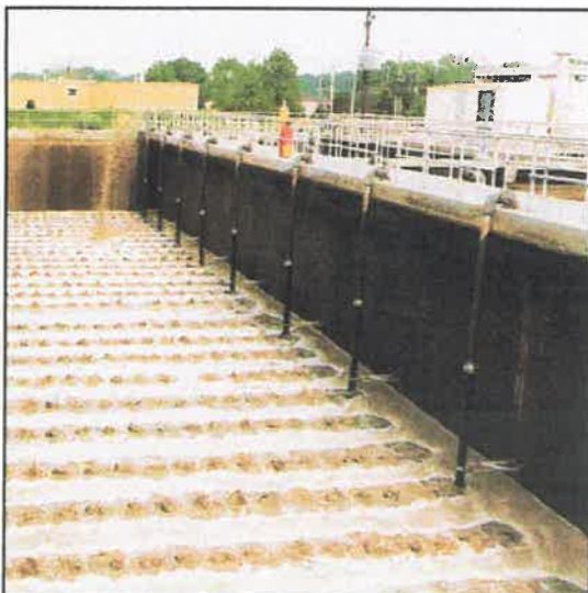
AERGRID™ Air Distribution Test
