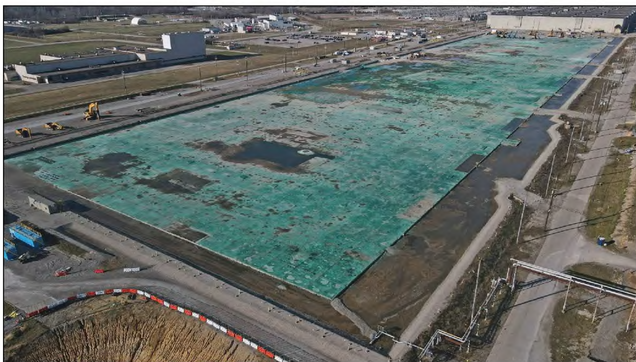
Figure 5. Aerial Photograph of the Condition of the Remaining Concrete Slab of the X-326 Process Building (as of November 2023)
