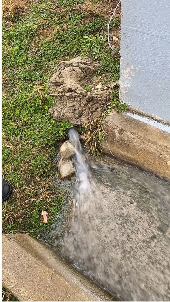
Figure 5. Still from a video. Image shows water flowing from a pipe located in the southwest corner of the facility building. Discharge was not continuous and was occurring in spurts indicating this may be a non-stormwater discharge.
