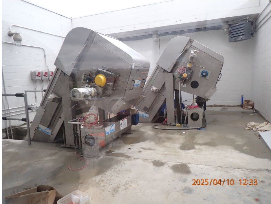
Figure 2. Two new mechanical fine screens. Photo taken 4/10/2025 by Whitney White. Pickaway Correctional Institution WWTP, NPDES #4PP00003.
