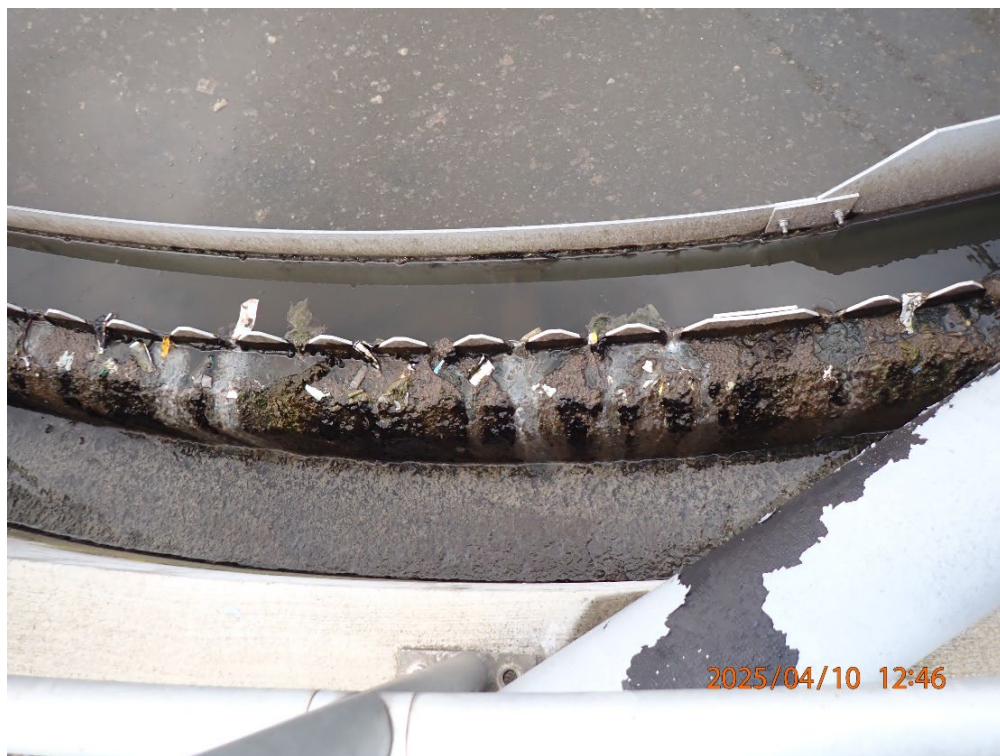
Figure 10. Sludge thickener weir. Photo taken 4/10/2025 by Whitney White. Pickaway Correctional Institution WWTP, NPDES #4PP00003.
