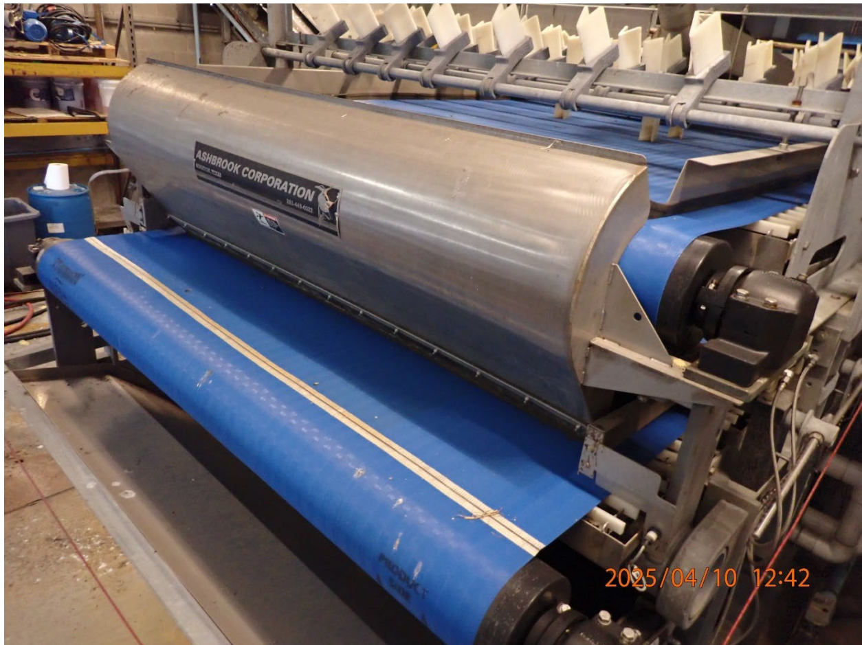
Figure 13. Belt filter press. Photo taken 4/10/2025 by Whitney White. Pickaway Correctional Institution WWTP, NPDES #4PP00003.
