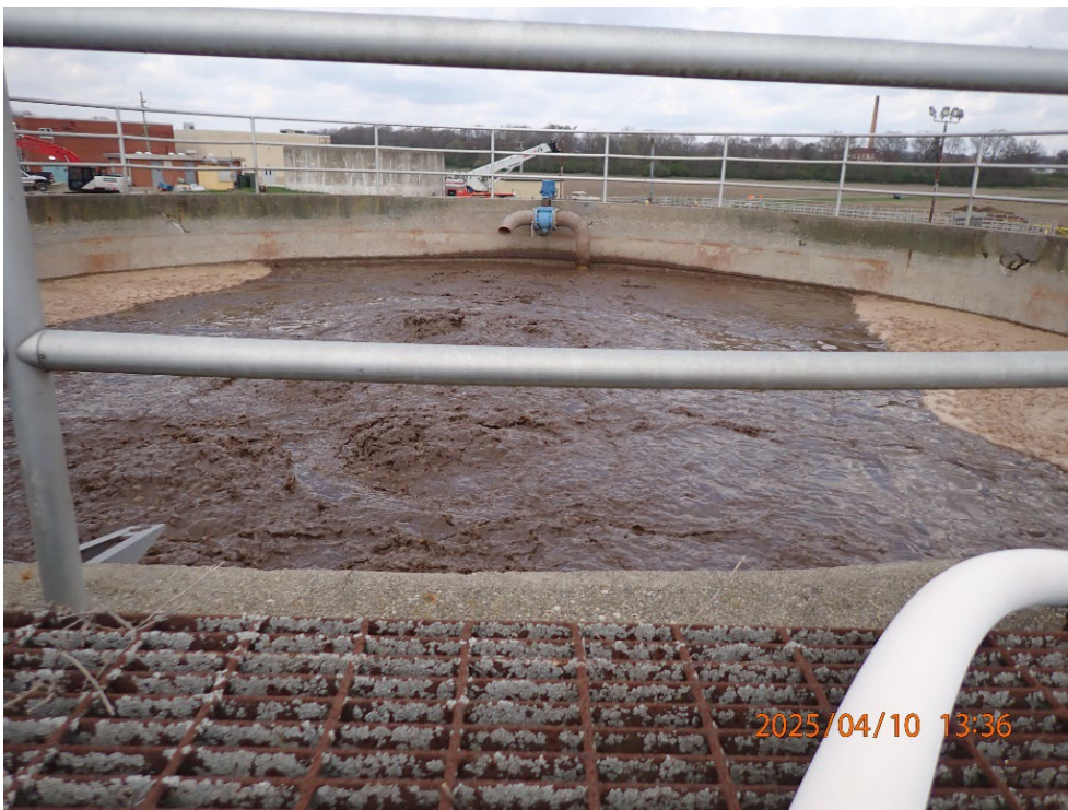
Figure 12. Aerated sludge holding tank. Photo taken 4/10/2025 by Whitney White. Pickaway Correctional Institution WWTP, NPDES #4PP00003.
