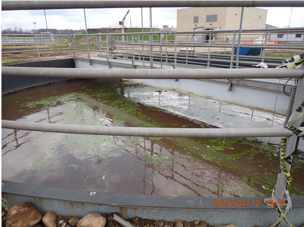
Figure 8. One of two anoxic tanks. Photo taken 4/10/2025 by Whitney White. Pickaway Correctional Institution WWTP, NPDES #4PP00003.
