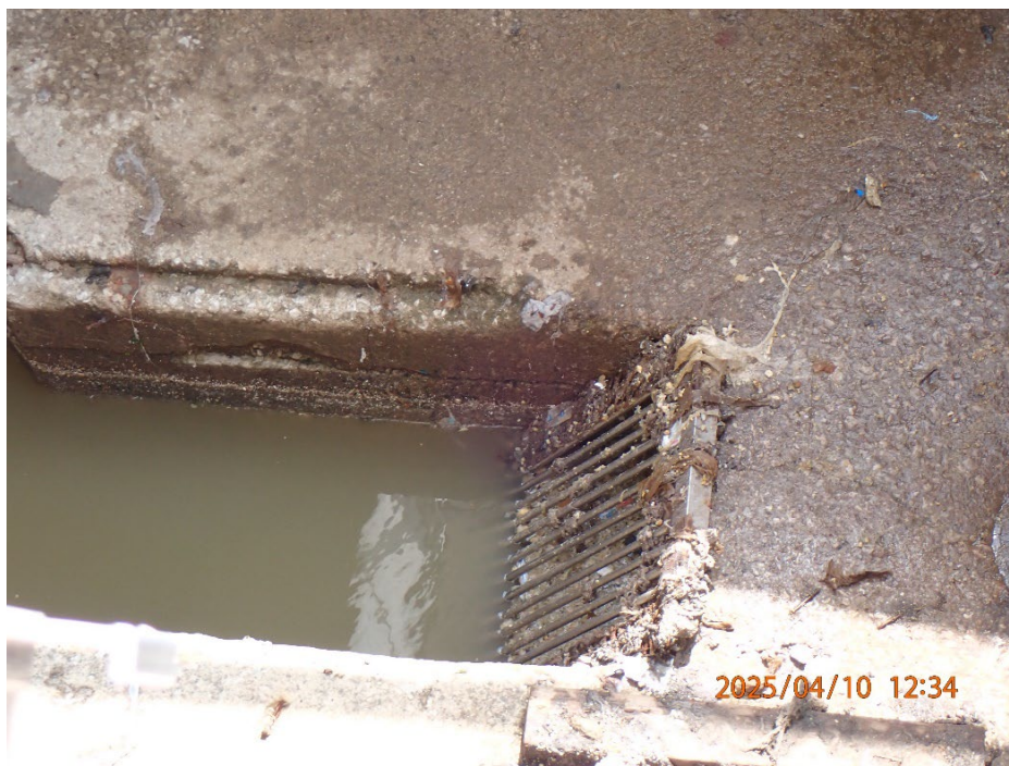
Figure 1. Influent bar screen. Photo taken 4/10/2025 by Whitney White. Pickaway Correctional Institute WWTP, NPDES #4PP00003.
