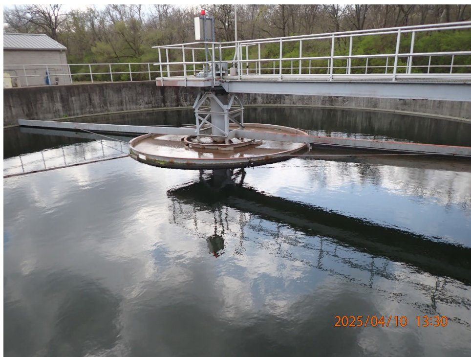
Figure 6. One of two clarifiers. Photo taken 4/10/2025 by Whitney White. Pickaway Correctional Institution WWTP, NPDES #4PP00003.
