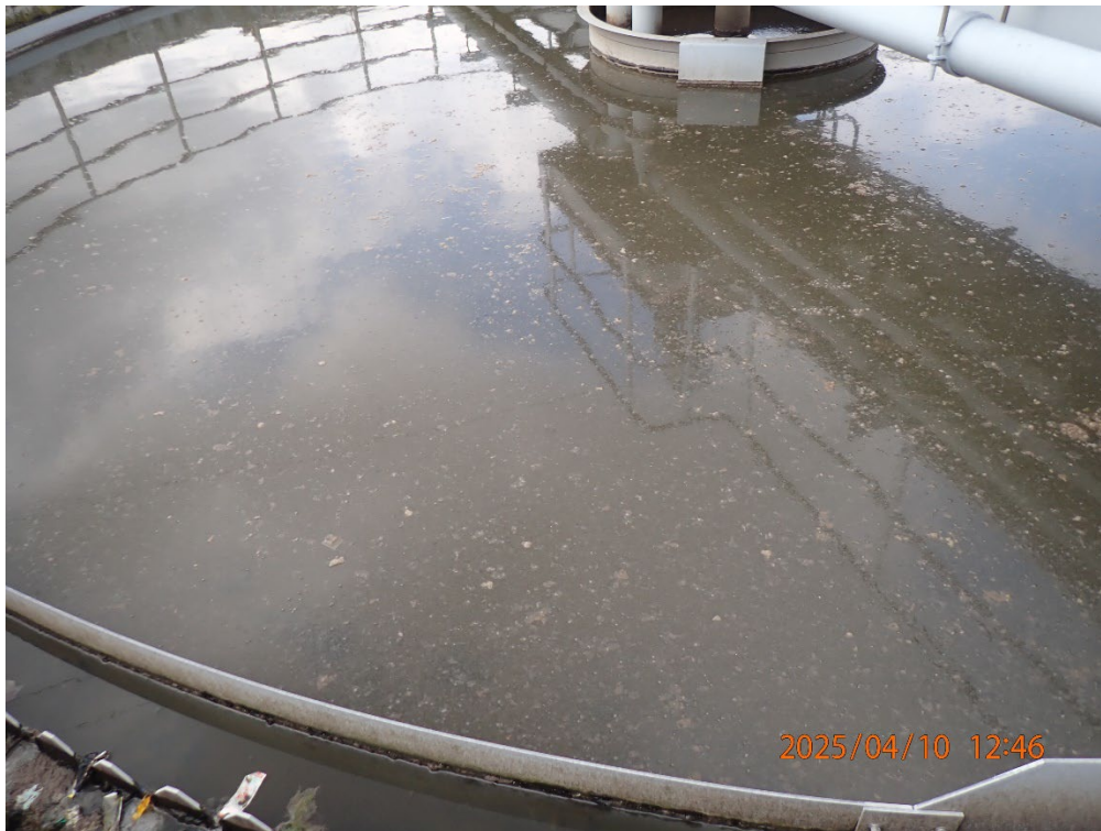
Figure 9. Sludge thickener. Photo taken 4/10/2025 by Whitney White. Pickaway Correctional Institution WWTP, NPDES #4PP00003.
