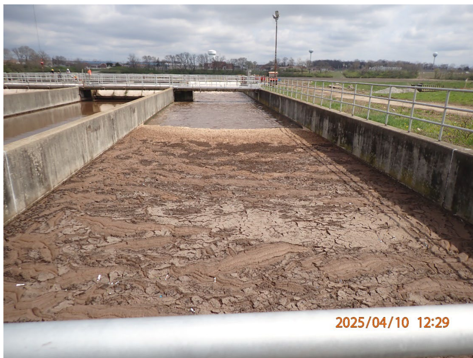
Figure 4. South oxidation ditch. Photo taken 4/10/2025 by Whitney White. Pickaway Correctional Institution WWTP, NPDES #4PP00003.
