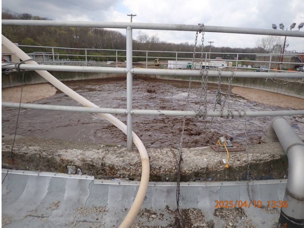
Figure 11. Aerobic digester. Photo taken 4/10/2025 by Whitney White. Pickaway Correctional Institution WWTP, NPDES #4PP00003.
